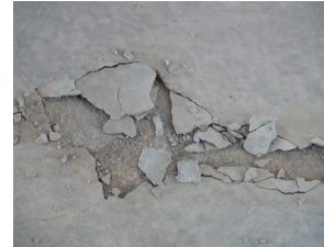
Delamination for repair
