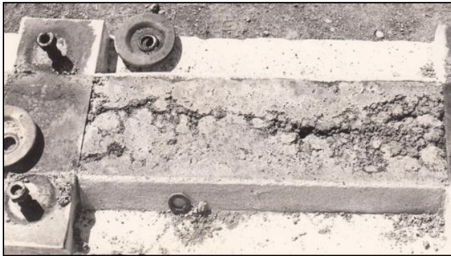
Compromised bearing area
