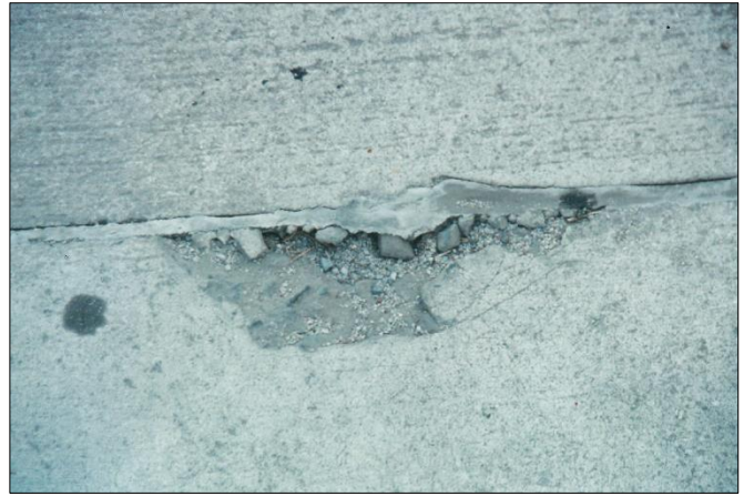
One sided construction joint failure
