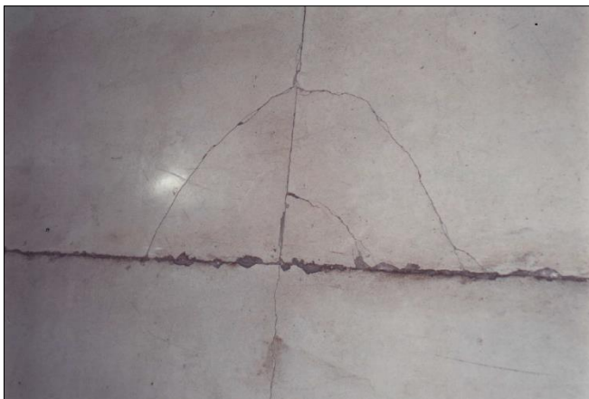
Undefined shutter edge with associated slab curling
