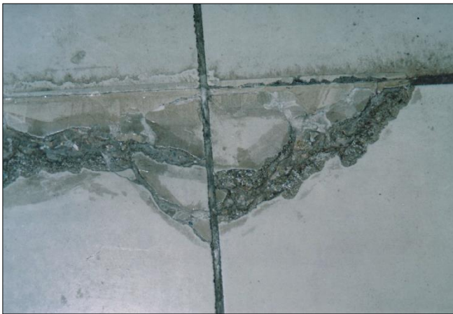
Failed joint with associated slab curling
