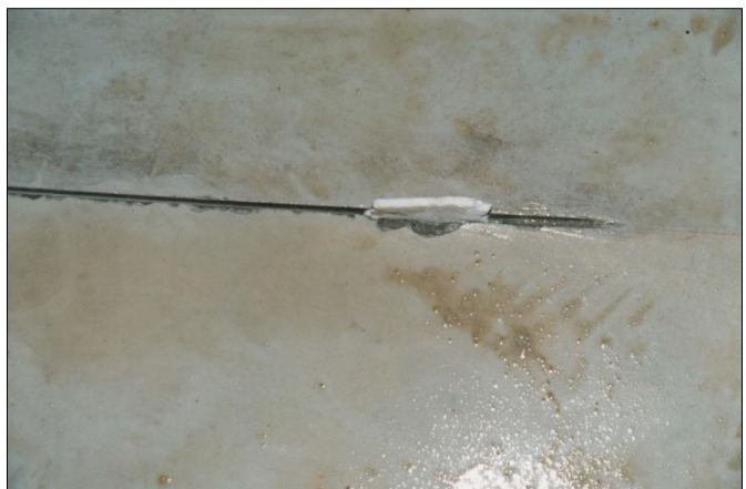
Poorly attempted repair
