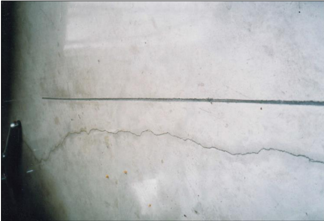
Cracking adjacent to construction joint
