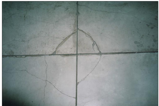
Misplaced saw cut with associated slab curling
