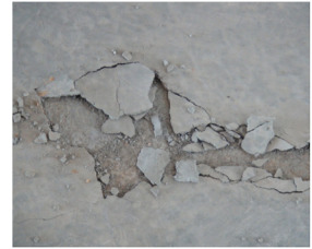
Delamination for repair
